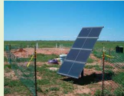
PV array to pump 2-3 gpm of water through a low-energy mulch bioreactor at Altus AFB in Texas
