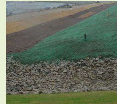
Rock-filled stormwater channels and erosion control blankets used for excavation and backfilling at former U.S. Navy landfill
