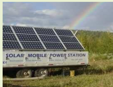
Portable PV system for 5-month SVE after oil pipeline break at Rocky Mountain House air base in Alberta, Canada
